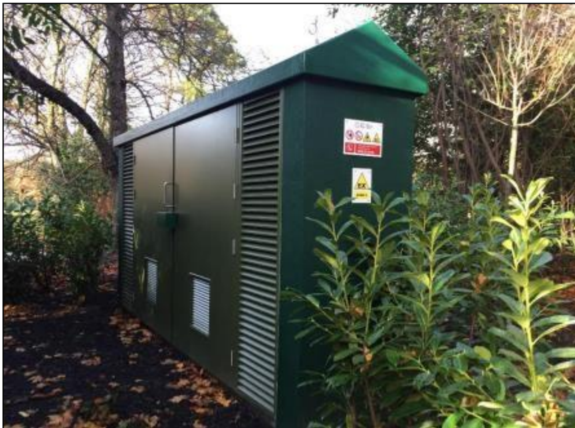
Figure 17.5: St. Stephens Green DRI – Custom Installation – Landscaped / GRP Enclosure.
